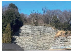
Grating crib work to protect houses from landslides (Wada area, Tama City)
